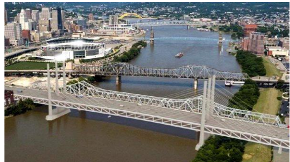
The Brent Spence Bridge, connecting Covington to Cincinnati, is in desperate need of rehabilitation. Certainly Americans would be better served by a federal government that took care of domestic infrastructure concerns first. Photo Credit: https://rb.gy/te3kid
